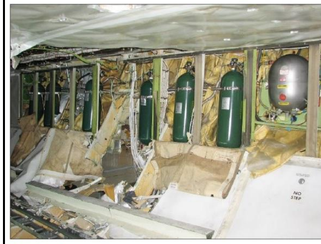
Figure 9: Forward cargo hold wall with remaining six oxygen cylinders
